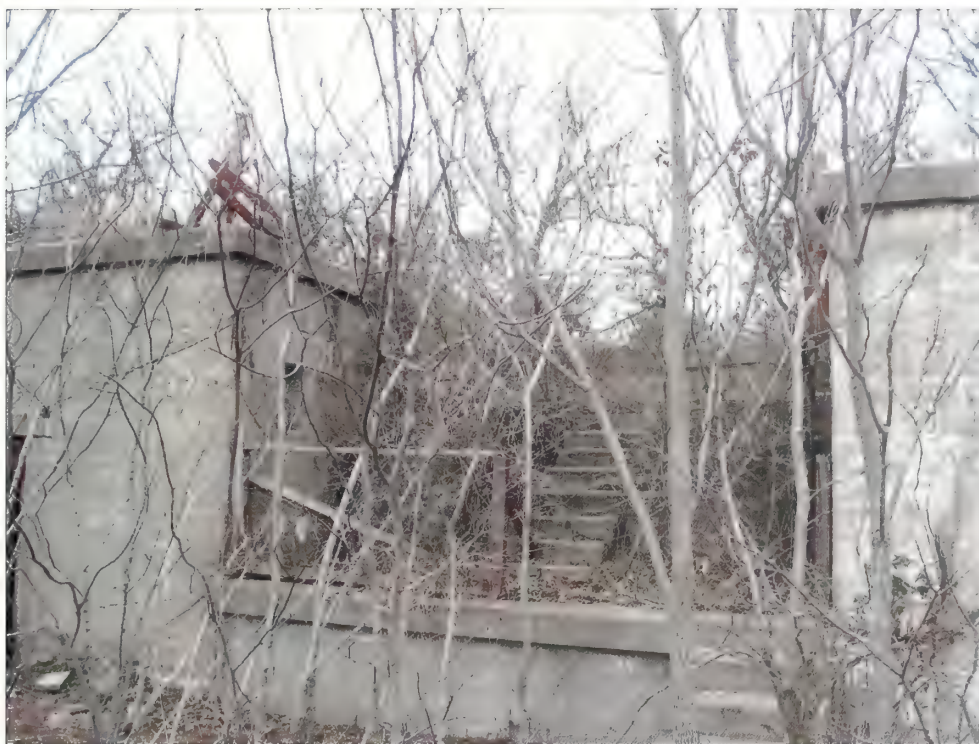
Figure 5.33. Wood guard panels at Battery Morris. The wood panels are not a historic feature and do not comply with safety codes due to the excessive space between the rails and cross brace. The wood guard panels should be removed and great care should be exercised not to damage the historic concrete structures removing fasteners that secured the wood to the concrete (Olmsted Center, January 2009).
